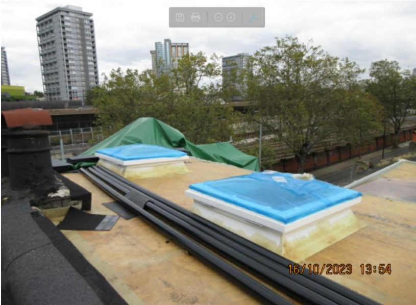
Photo looking northeast at roof level and photo looking east towards no.66 at roof level
